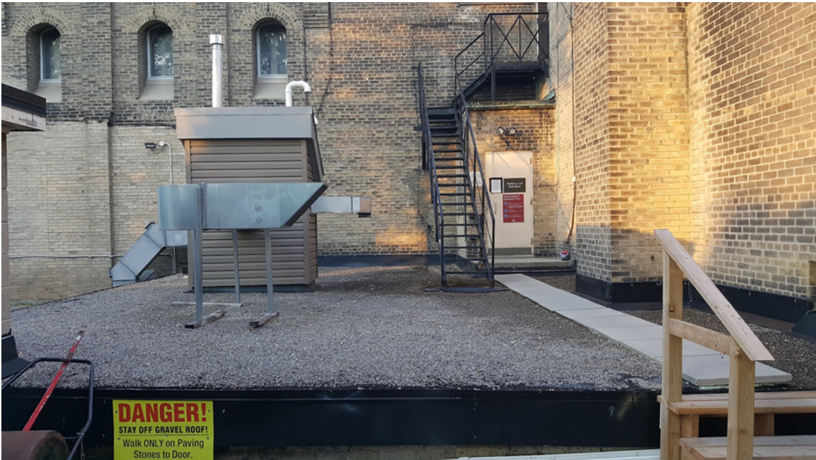
Boiler room roof with kitchen air handling equipment and fire escape complicating re-roofing.
