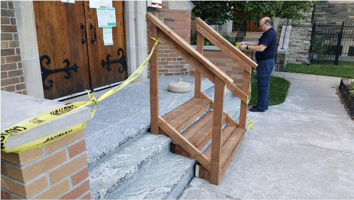
Jewitt steps with granite cladding, temporary code-compliant steps, Jim
